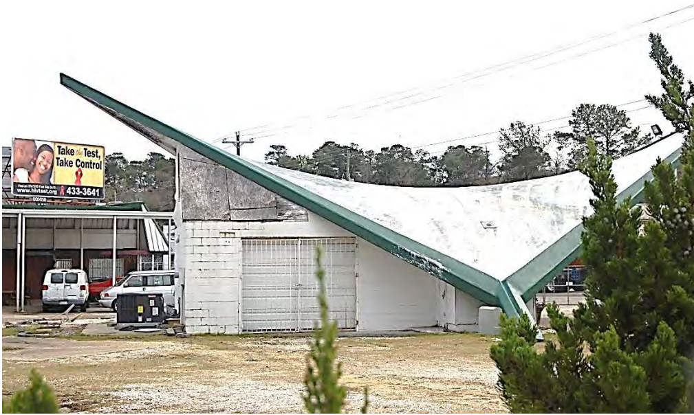
Plate 35. Pam-Oil Gas Station, North Elevation, Looking East. (Plywood Roof Visible Above Garage Door.)
