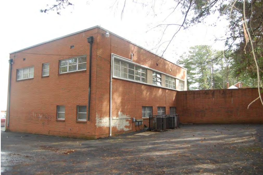
Plate 8. Stewart Building, Side (West) and Rear (North) Elevations and Retaining Wall, Looking Southeast.
